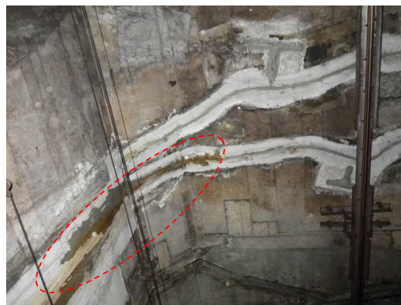
(b) Recurrence of water leak
